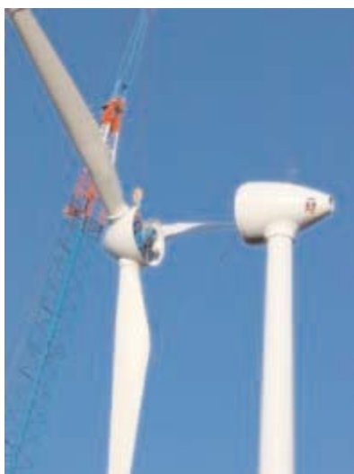
Figure 6. The installation of the blades and hub on one of the 12 turbines.
